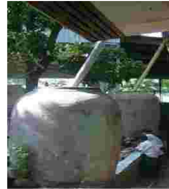
Rainwater harvesting system
